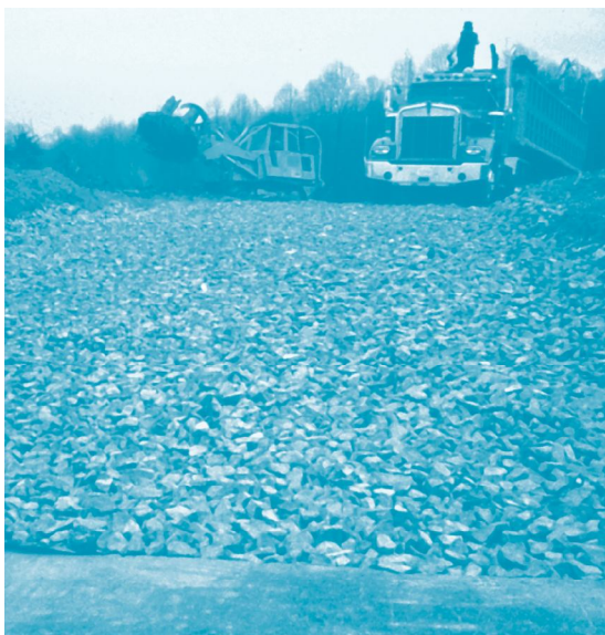
Large, heavy rocks prevent dirt from being tracked onto streets in this properly maintained construction entrance. Dirt on the streets will eventually end up in storm drains.
