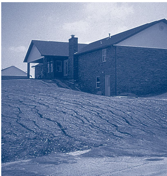
Improperly maintained slopes result in runoff and erosion.
